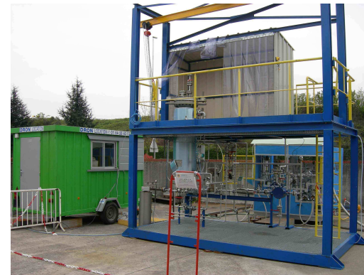
THT capture with activated charcoal 1,5 MW – 12 bar (tested at 70 bar)
