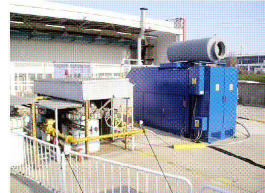
Cogeneration 400 kWe Turbin helicopter equipped with silencer
